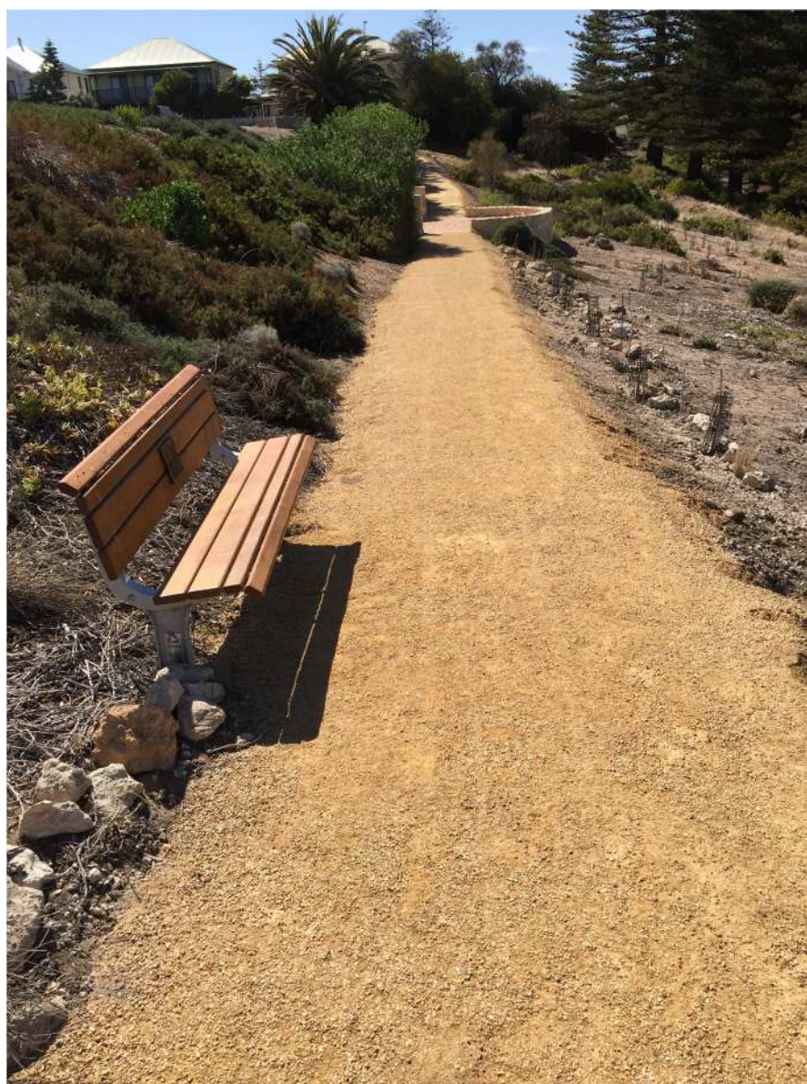
Safer path as constructed by Alexandrina Council to this area. They will also construct the wooden seats on the stone supports.
